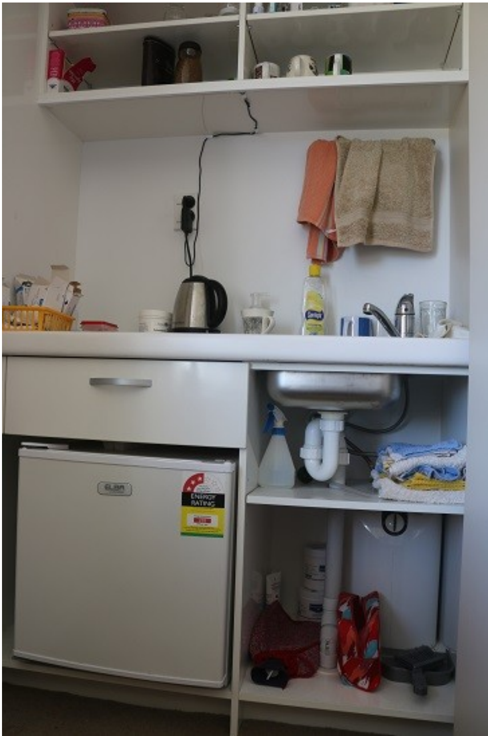
Bar refrigerator in ensuite kitchenette. Note push-through water heater.
