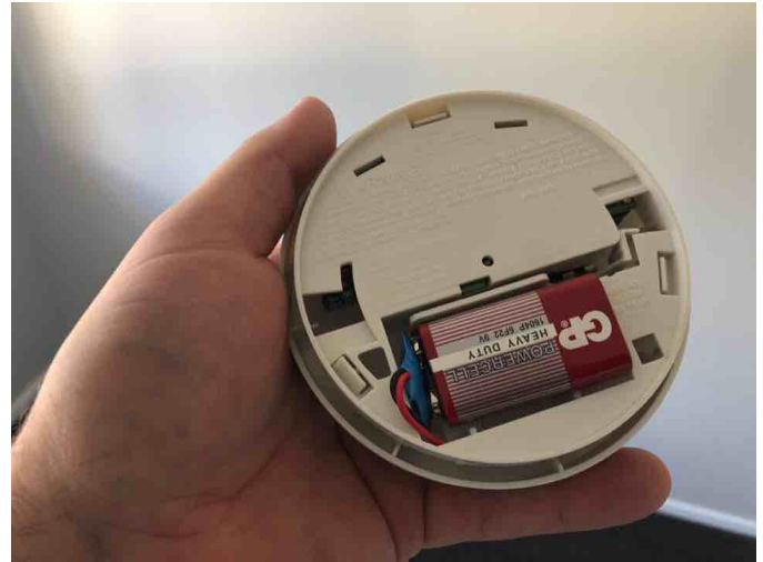
Qualifying Photoelectric smoke alarm noted and tested. Meets the Healthy Home standard. Replacement date 2025
