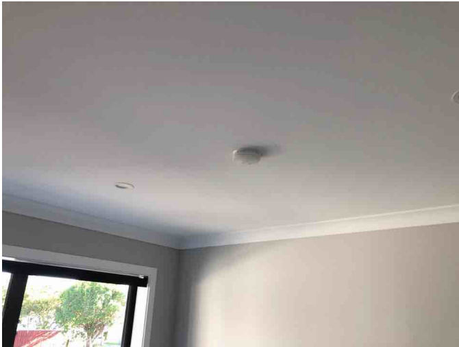
Smoke alarm located within bedroom: 1
