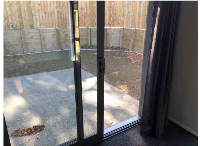
The openable door complies with the 5% ventilation requirement for this room and section 21 of the Healthy Homes Standard.
